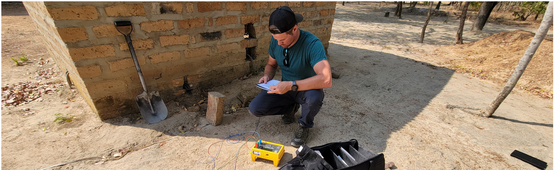
above: Tim testing existing electrical conditions on site (photo: Ben Shinabery - Itezhi Tezhi, Zambia)
